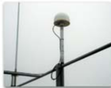
High-precision Columbia sensors are placed in pairs in opposite corners of the top floor of each building in the study. This allows researchers to detect the motions of the structures along lateral perpendicular axes, as well as twisting motions. An ultrasonic anemometer and Global Positioning System antenna, shown above, are also utilized in the study. Before installing any hardware, however, the Notre Dame team spent two years calibrating the sensors to the urban environment in order to assure reliable measurements.
