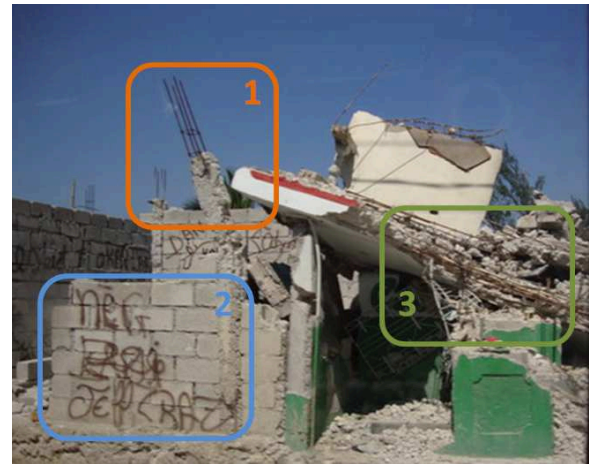
Fig. 6. While 3 professionals achieved agreements on the Column damage in Area 1 and Wall damage in Area 2, they took different positions on whether there was a Beam damage in Area 3. (Professionals were not required to draw frames while tagging photos)
