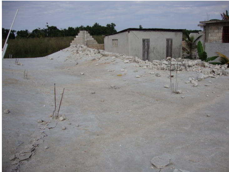
Figure 4.12. Strong Consensus Type 2: Building entirely collapsed.
