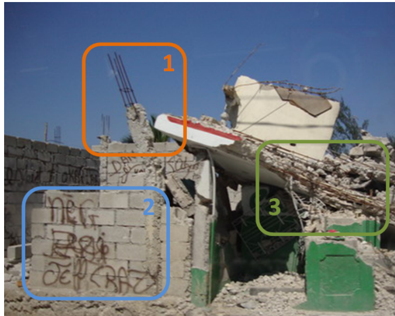
Figure 4.18. While 3 Professionals achieved agreements on the Column damage in Area 1 and Wall damage in Area 2, they took different positions on whether there was a Beam damage in Area 3. (Professionals were not required to draw frames while tagging photos.)
