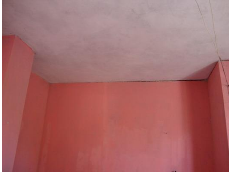
Figure 4.11. Strong Consensus Type 1: Building has no significant damage
