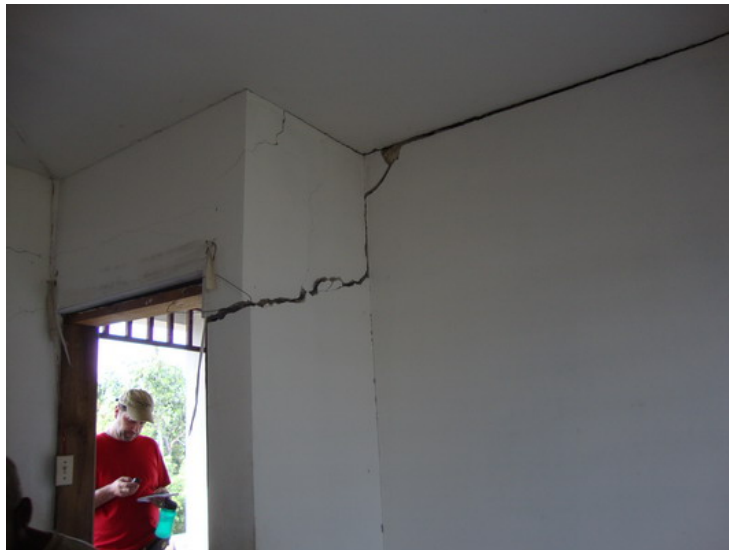
Figure 4.15. Weak Consensus Type 1: Major damage at column and minor damage on wall.
