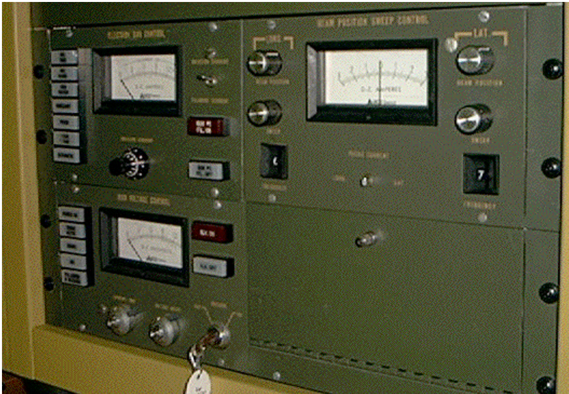
Figure 2: HVPS Controls High Voltage and Beam Control sitting on top of the CV14 power supply.
