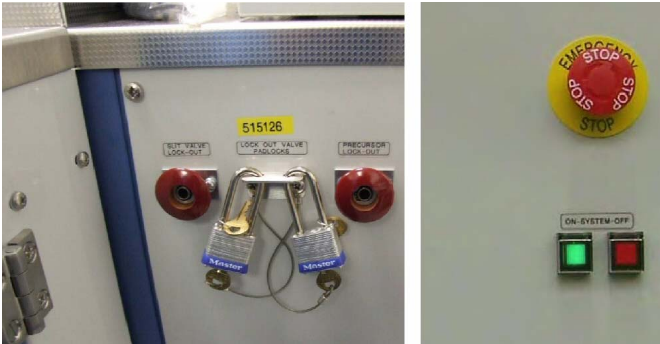
Figure 4-1 System control panel
