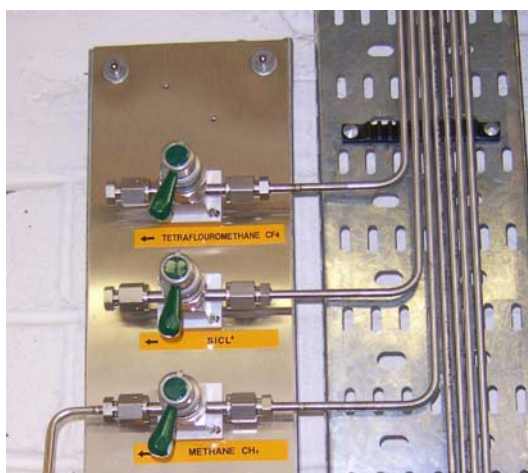
Figure 10-16 Gas supply point-of-use valves
