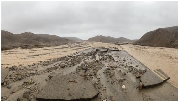
Photo of flood damage at Mud Canyon Road in Death Valley National Park, California, from August 2022. On August 5, 2022, the park received 1.70 inches of rain — an all-time 24-hour rainfall record for the area. (National Park Service)
