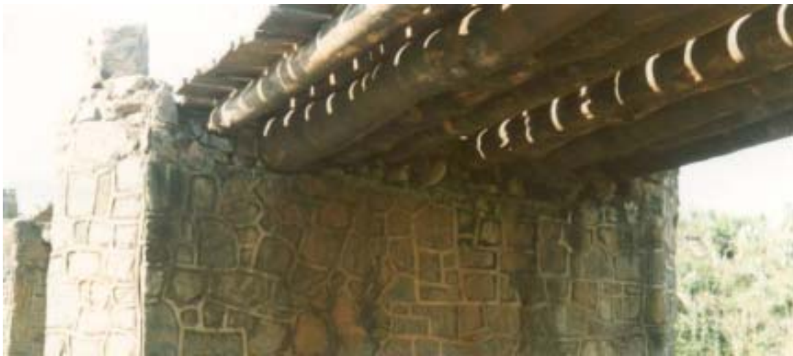
Timber log bridge supported on masonry abutments and piers. Note the way in which the masonry has been built up to support the stringer logs of different sizes and also between the logs to locate them in position.
