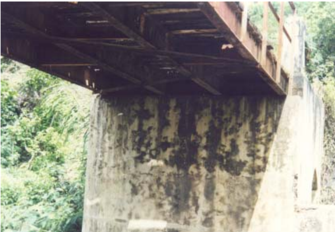
View of the underside of the bridge showing the 4 I-section steel beams. Note the cross-bracing that is used to prevent twisting of the beams under load
