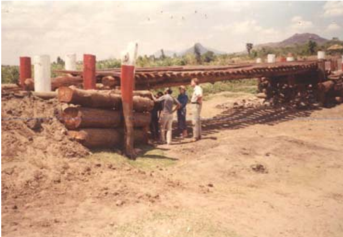
Timber log bridge supported on timber crib abutments and with timber log wing walls
