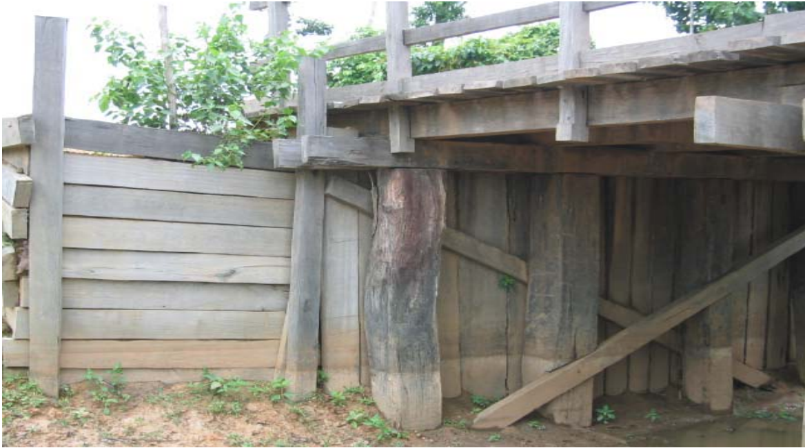
Detail of sawn timber abutment with sill supported by 3 posts. Note the timber behind the abutment and the wing wall to protect against erosion of the bank.
