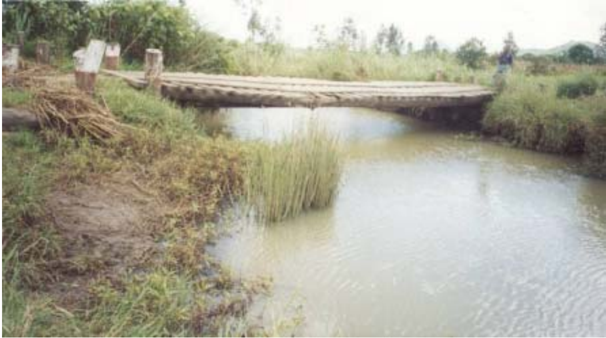
Figure 3.3: 13m Span Log Bridge in Malawi (Note the running boards on the deck for vehicles)
