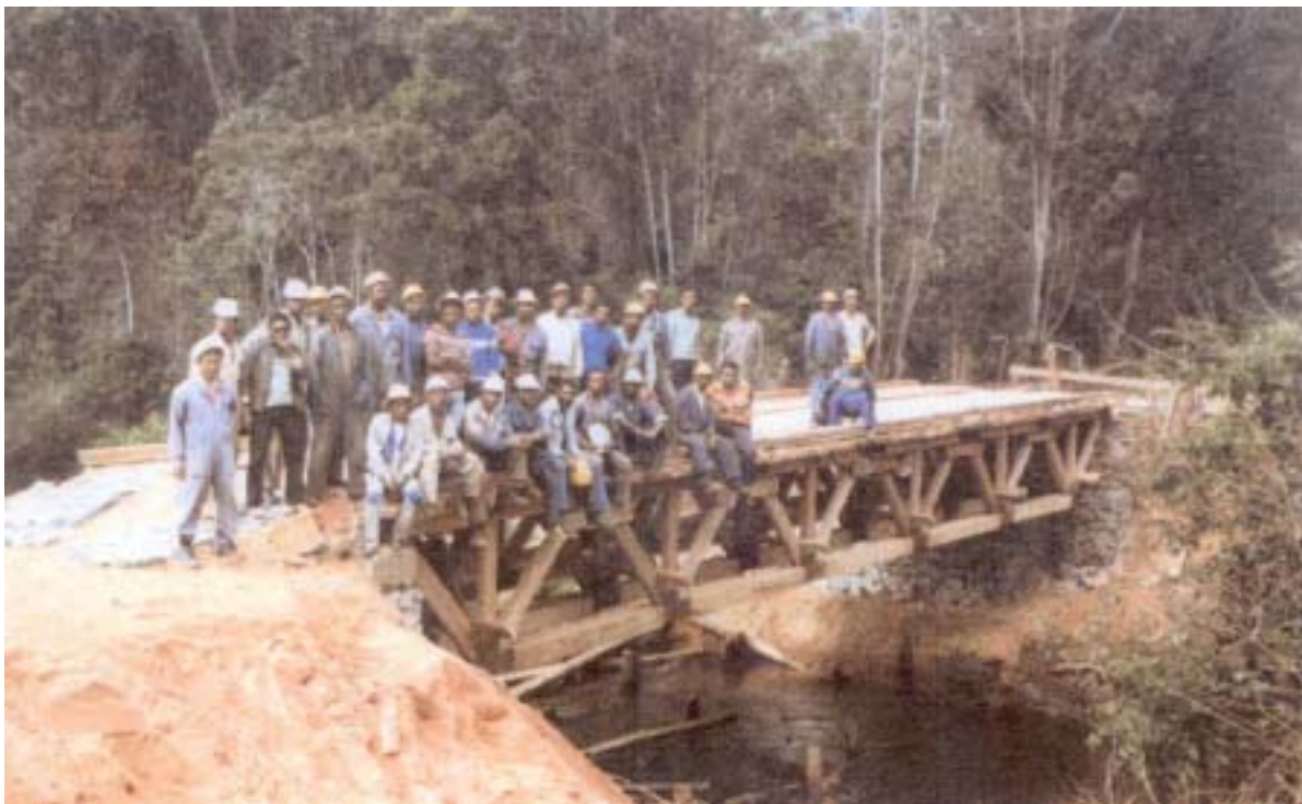
Figure 3.9: A Modular Timber Truss Bridge Developed by UNIDO and TRADA. The 18m span bridge in Madagascar was erected in 4 days on prepared abutments
