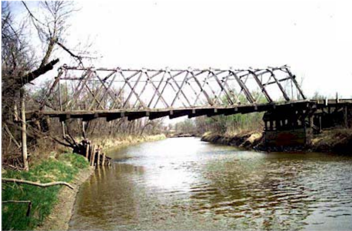
A 'parallel chord' truss bridge of about 20m span constructed in Canada. This bridge was 62 years old at the time of the photograph.
