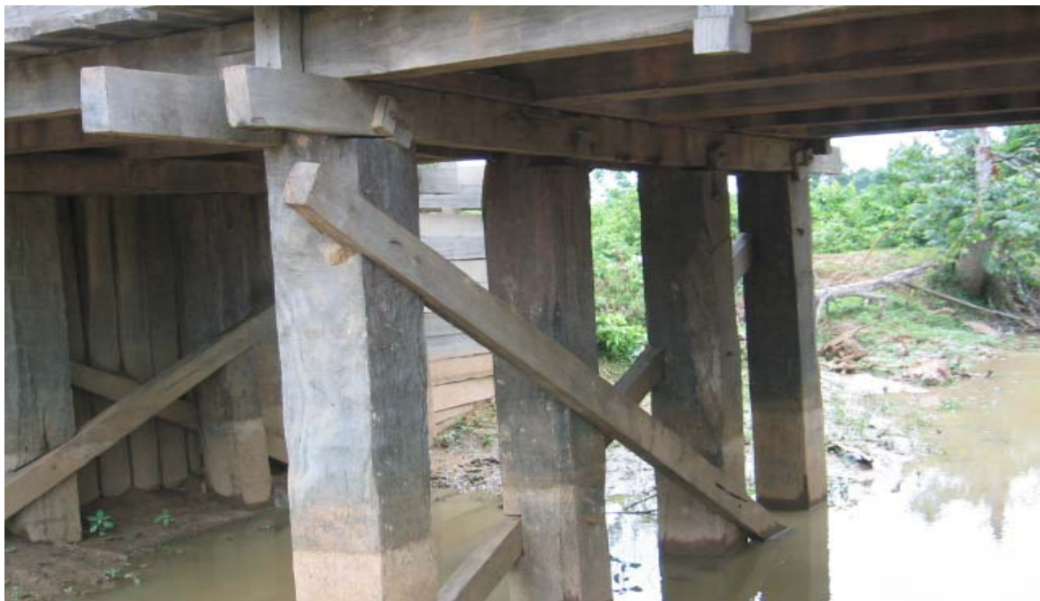
Detail of pier support of timber stringers. Note the butt joint of stringers with 2 cross-beams supporting the ends of the stringers.
