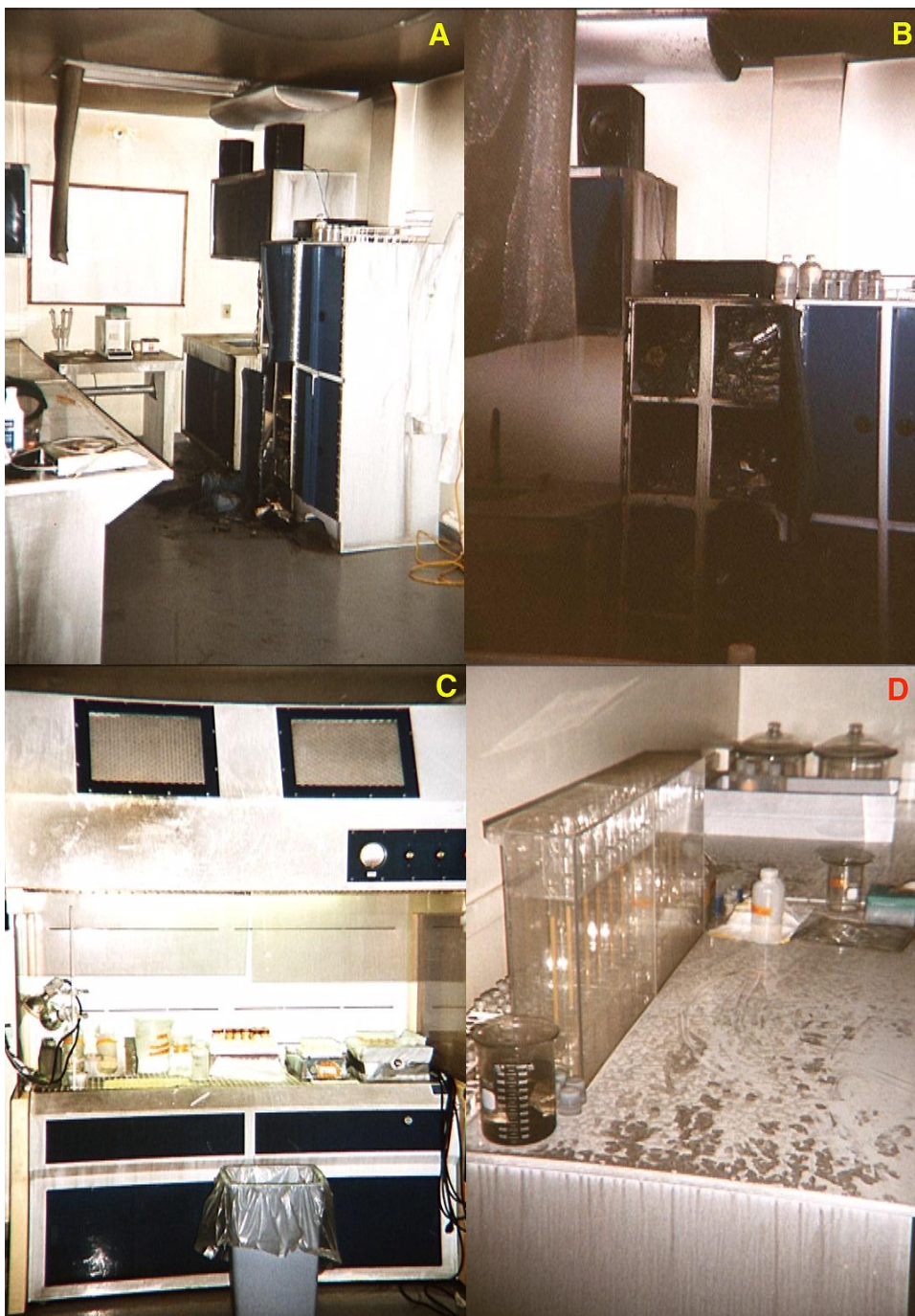
FIGURE 2: Damage that resulted from the 1997 fire in the ICP-MS sample preparation laboratory, 112F Cushing Hall.
