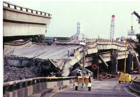
Collapsed double-decked Cypress freeway in Oakland after the 1989 Loma Prieta earthquake.
