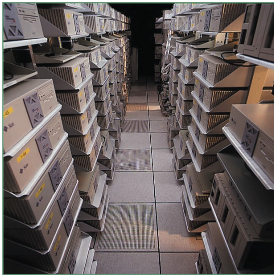
Figure 4. 100-node 200-CPU cluster. Key design points include extreme symmetry, internal disks, no people, no monitors, and no visible cables.
