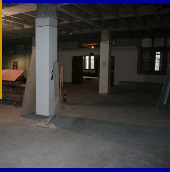
LEFT: A look at the false floors of the old Stacks, deconstructed.
