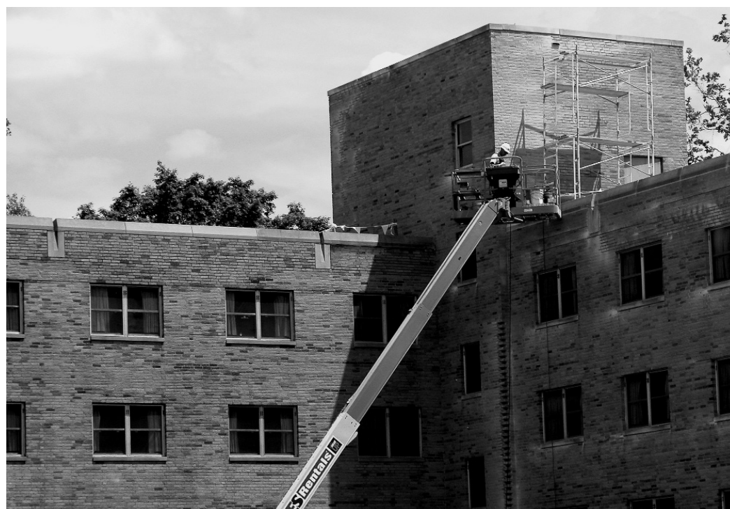
Workers at Stanford Hall repair parapet and prepare to replace the roof. Nearby, another construction crew continues gutting the Student Health Center. Just a few yards to the north of the two buildings, a project to extend chilled water mains that support the campus air conditioning system has created a deep ditch that runs along Holy Cross Drive. Other on-campus summer roofing projects are being undertaken at Fitzpatrick Hall, Galvin Life Science Center, Lobund Laboratory, the Loftus Center, and the Morris Inn, where exterior repairs also are under way. Across from the Morris Inn, the front yard of McKenna Hall has been torn up so the tunnel running between the two buildings can be waterproofed. Renovations also are being made to the Decio Hall exterior walls, and on Dillon Hall. Off campus, the former Logan Center is being razed to make way for the straightening of Edison Road. ND Works staff photo.
