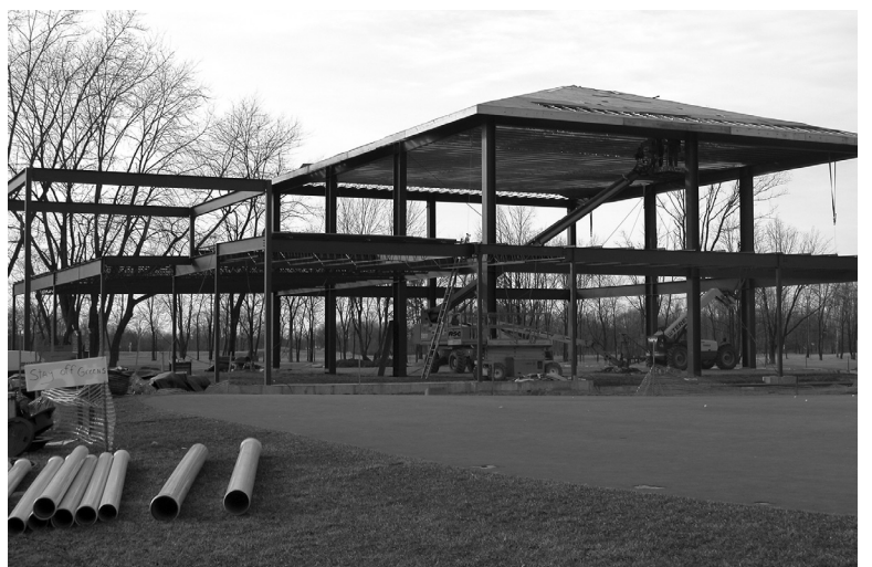
This indoor practice facility under construction at the Warren Golf Course will house the men's and women's golf teams, their coaches, and cutting-edge practice facilities. ND Works staff photo.
