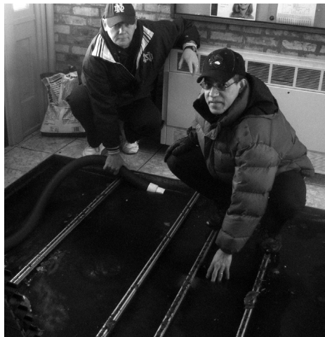
Michael Crabtree, left, and Virjilio Eschevarria, washer/shampoos for Building Services, became "water pumpers" when the recent cold snap caused a burst pipe in the Main Building. Photo by Alan Bigger.
