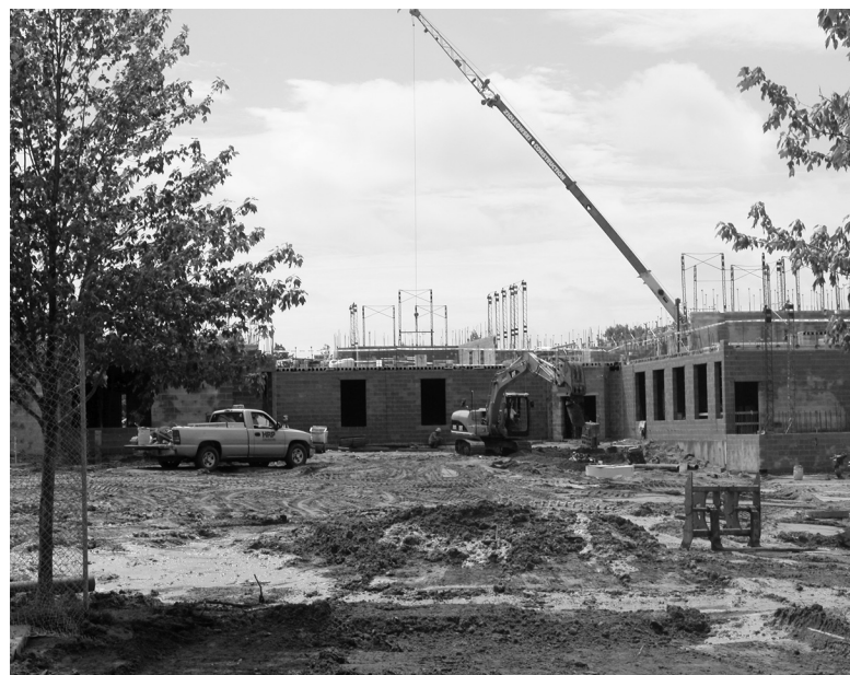
A busy summer of construction has given shape to Duncan Hall, a new men’s residence west of McGlinn Hall on the University’s West Quad. ND Works staff photo
