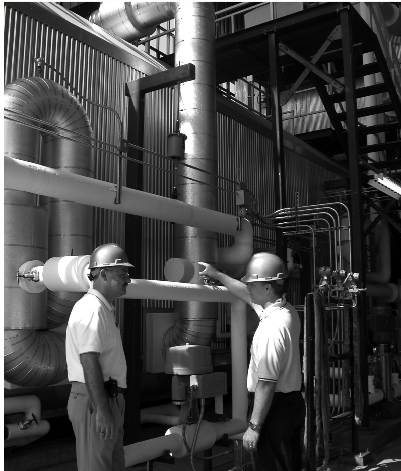
Craig Fritts, right, a mechanical engineer who oversees the commissioning of Boiler No. 6, discusses the process with project manager Mark Hummel. ND Works staff photo
