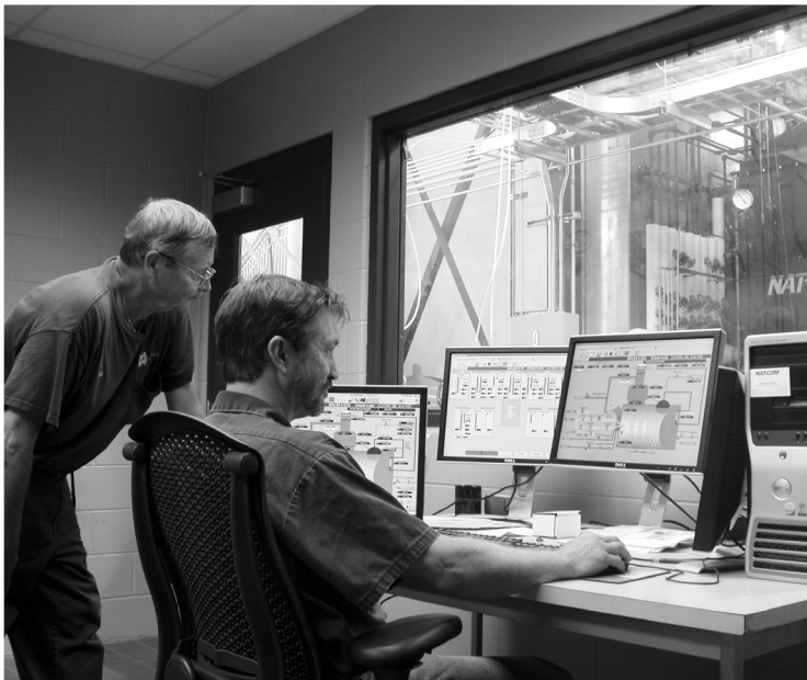
In the control room of the new boiler facility, shift supervisor Larry Maitlang, seated, familiarizes mechanic Mike Olmstead with the Power Plant’s new computerized distributed control system. ND Works staff photo
