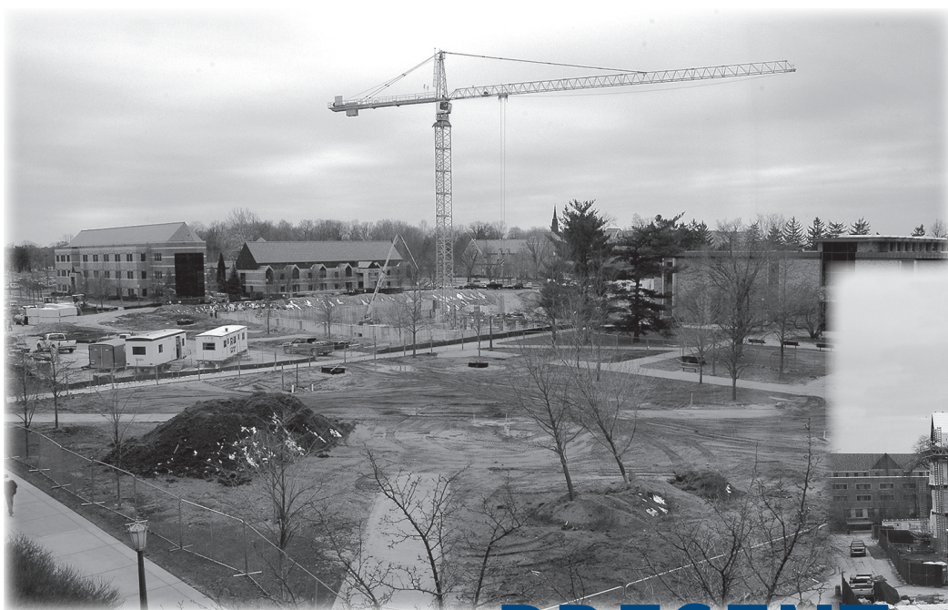
Construction of Stinson-Remick Hall, above, and the 85,000 square-foot Law School classroom/office addition, at right, will fill in some of the last remaining frontage on Notre Dame Ave. Photos by Carol C. Bradley.
