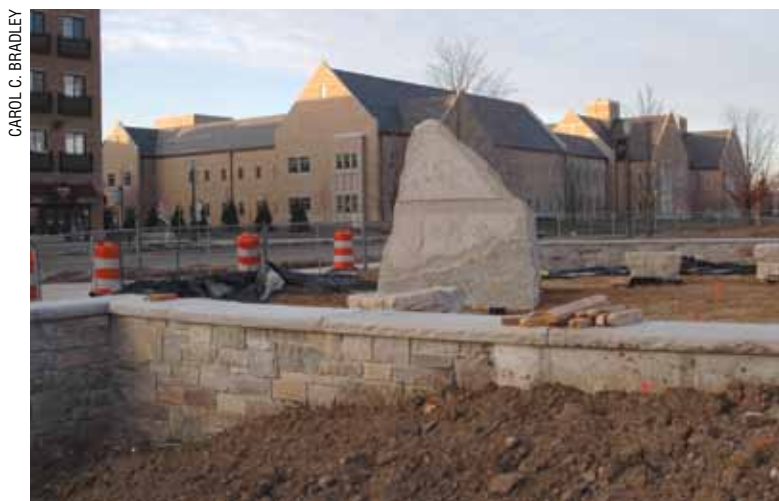
A new entry plaza at the southeast corner of the Irish Green includes a stone seating wall and new signage.
