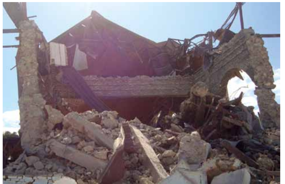
At top, Rue la Croix in Léogâne shows the extent of the devastation after the Jan. 12 earthquake in Haiti.
